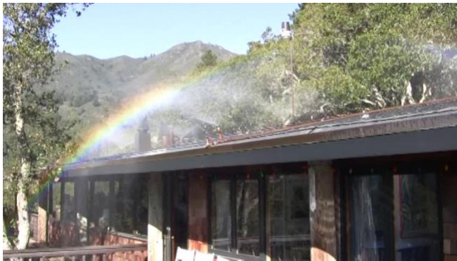
Figure 1. Example of an external sprinkler system for wildfire defense installed on a rooftop. Image courtesy of Steve Quarles.
